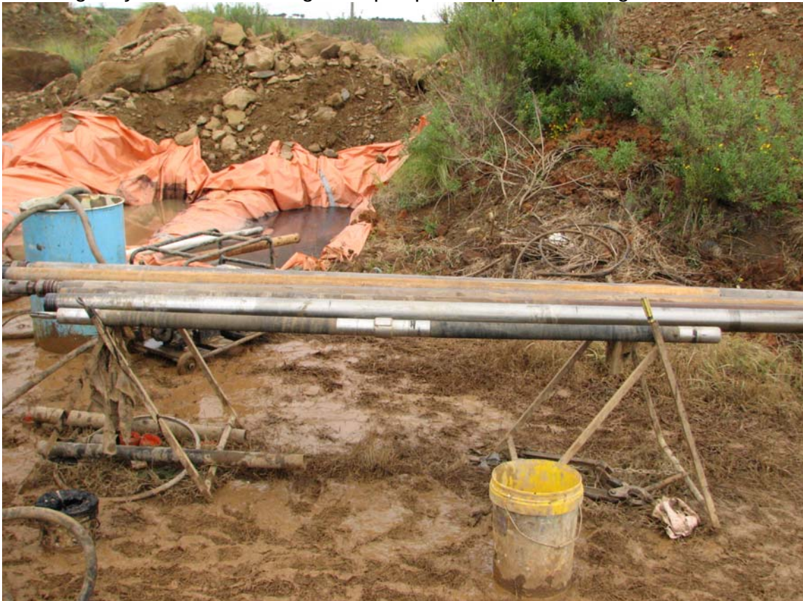
Packer on rack with pump and 200 litre water tank at rear
